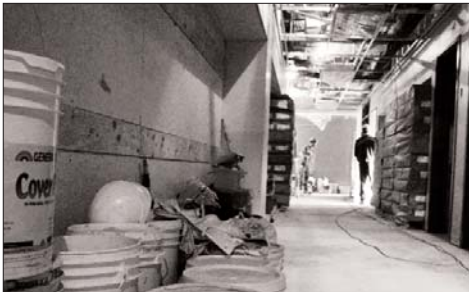
Amico workers finish up some electrical work in the new schools basement. The basement contains two new classrooms, a lounge, bathrooms and office space.
