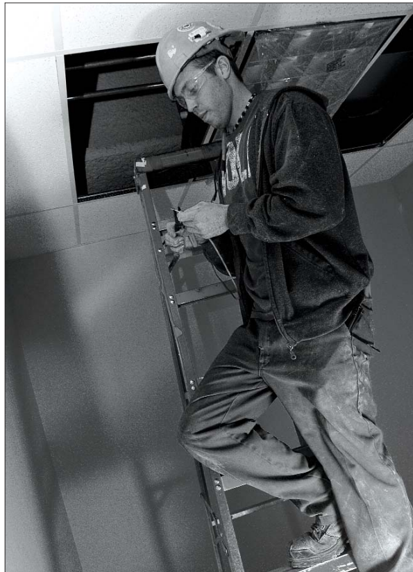
Electrician Kent Hergott works on the wiring in the basement classroom March, 5 2010 at the future school site for the St. Clair journalism program.
