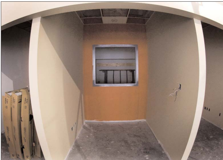
New editing studios are under construction along the back wall of the newsroom. These stations will allow students to edit their TV broadcast assignments.
