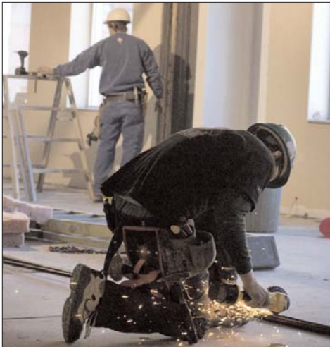
Vince Vitales cuts through metal rods while John Carmichael finishes framing a door in the new journalism building.
